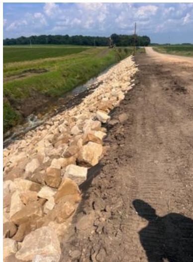
Left: reinforced bank with rip rap rock to help reduce bank sloughing and erosion issues. Right: Completed culvert replacement with reinforced ditch banks.
